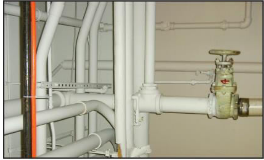
Piping and plumbing systems
